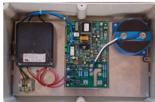
Heavy Duty power unit in Safe Area enclosure
