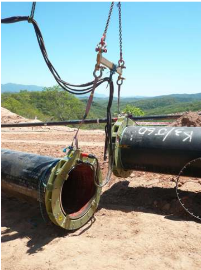
SHG used to power typical closed coil used for welding pre-heating
