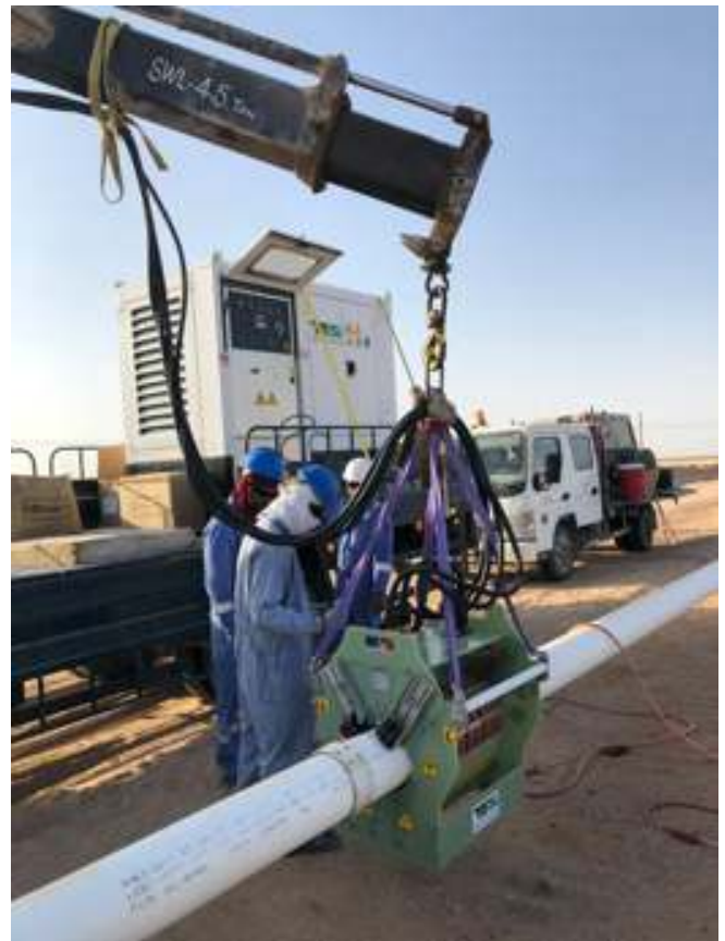
SHG used to power typical closed coil used for coating pre-heating
